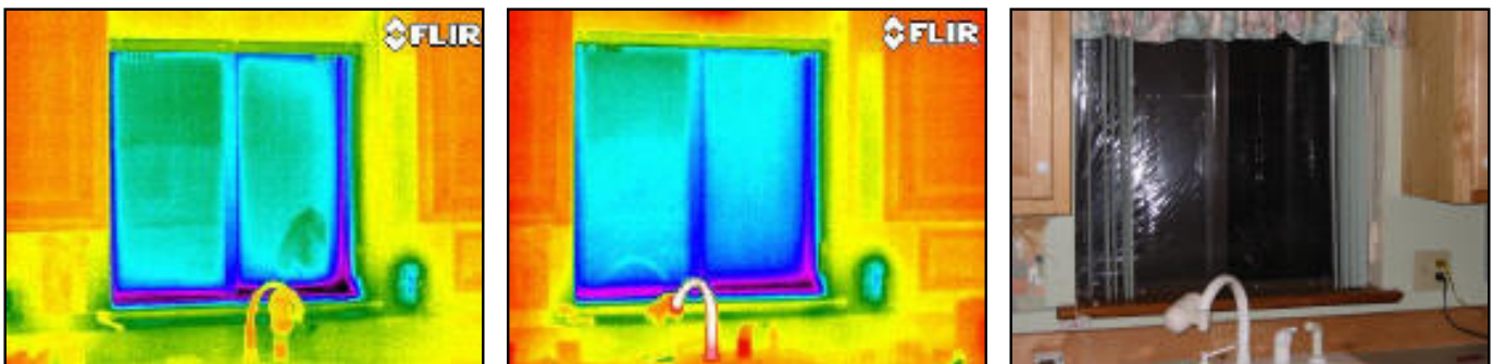
Window before and after application of plastic film (also note air leakage through the socket at right)
